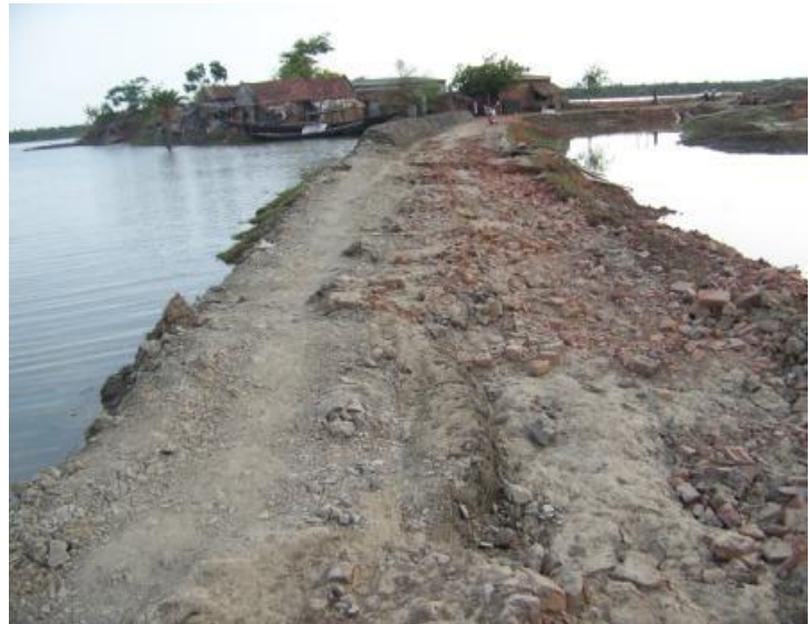
Photo: Damaged road in Koyra
